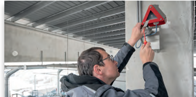
Assembly work of a GROMA Series 5A system in a recycling plant (Image: GROMA 247 / Tech2B)
