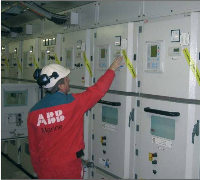
Picture 2: Medium-voltage switchgear monitored by fixed pyrometers
