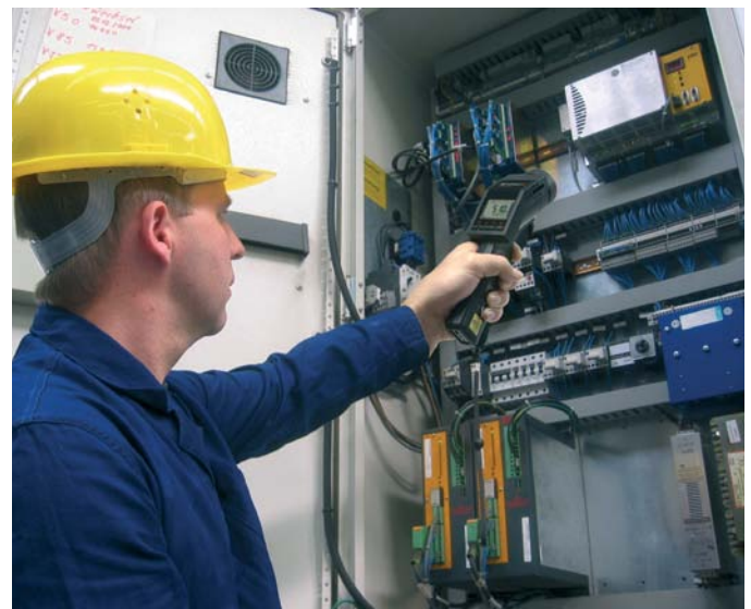
Picture 1: Temperature measurements on stressed components in a switch cabinet using the optris LaserSight LS
